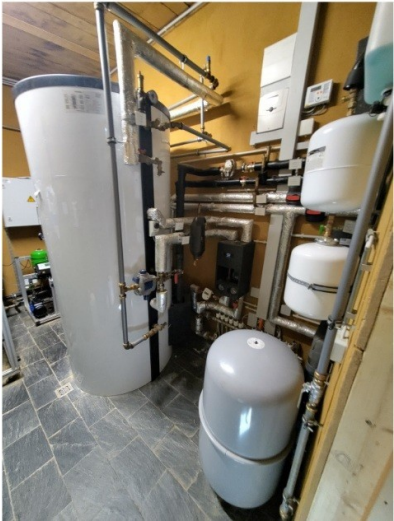
Treatment installation, EuroSolar photograph [E, p. 9].
